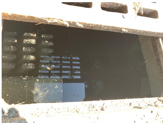
CB – 1 (Catch Basin)
