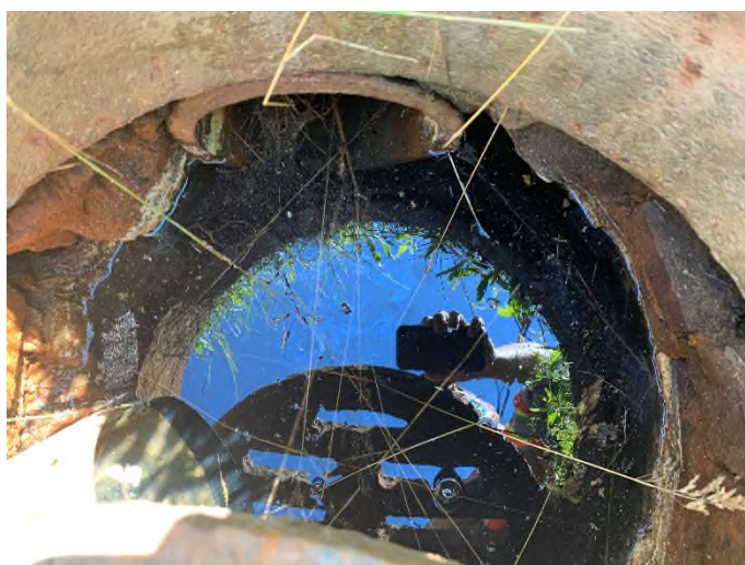
CB - 2 (Catch Basin)
