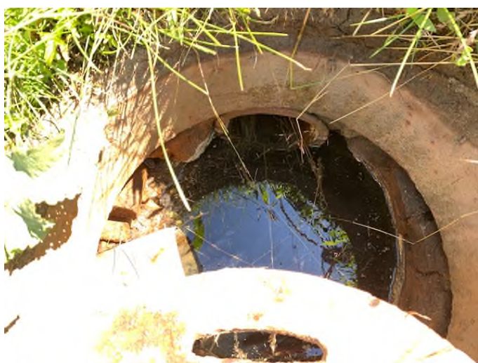
CB – 2 (Catch Basin)
