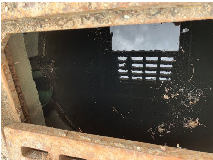
CB – 1 (Catch Basin)
