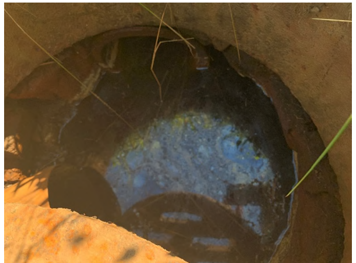
CB – 2 (Catch Basin)
