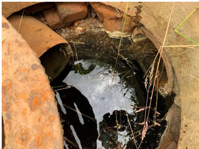
CB – 2 (Catch Basin)
