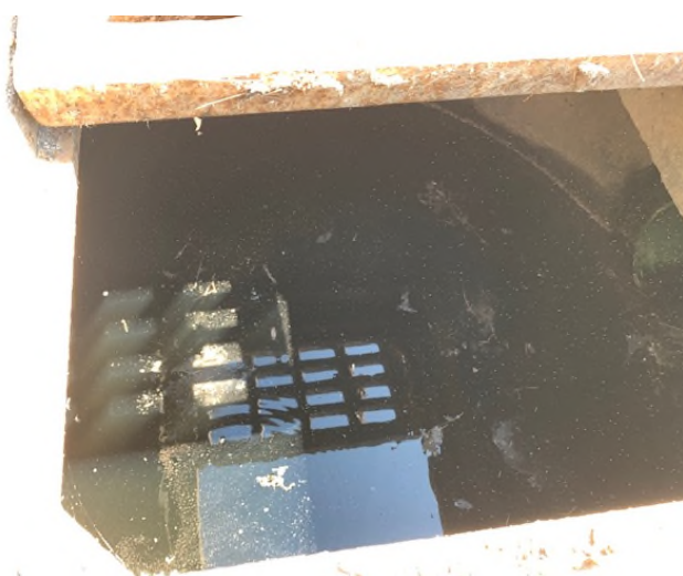
CB – 1 (Catch Basin)
