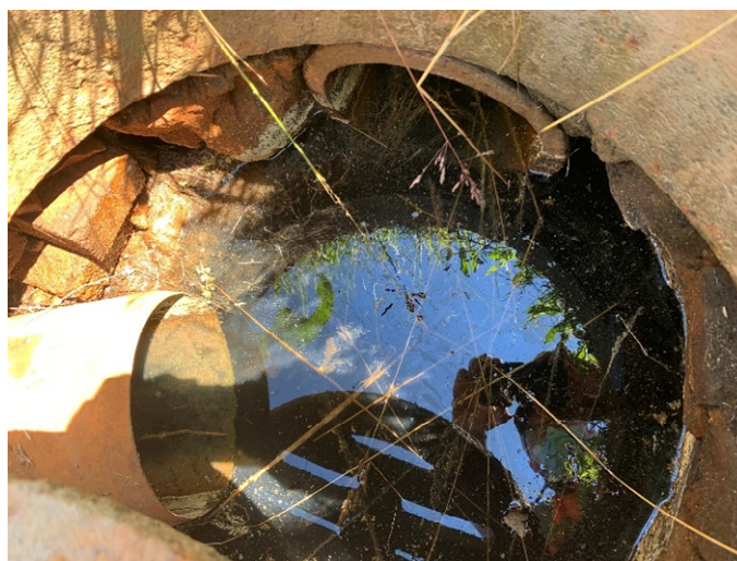
CB – 2 (Catch Basin)
