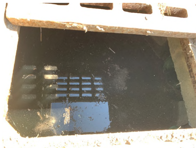
CB - 1 (Catch Basin)
