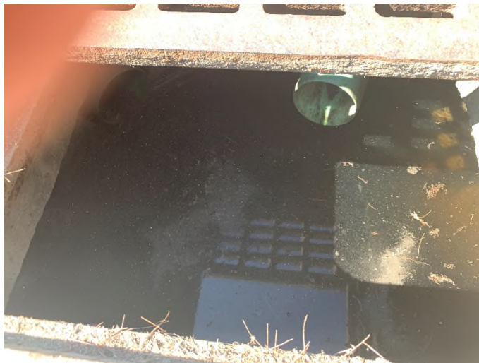
CB – 1 (Catch Basin)
